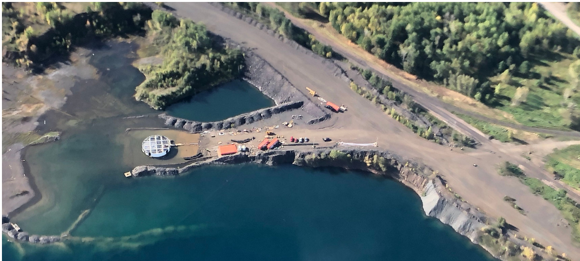
Figure 3.10: Aerial picture of the CHIPS-5 construction site facing south. The Wentworth 2W pit is in the lower half of the image, with the part built CHIPS-5 detector visible at the bottom of the earthen construction ramp. The two white shore huts can be seen halfway up the ramp.
